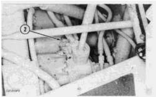
Compensator Valve On Pump
