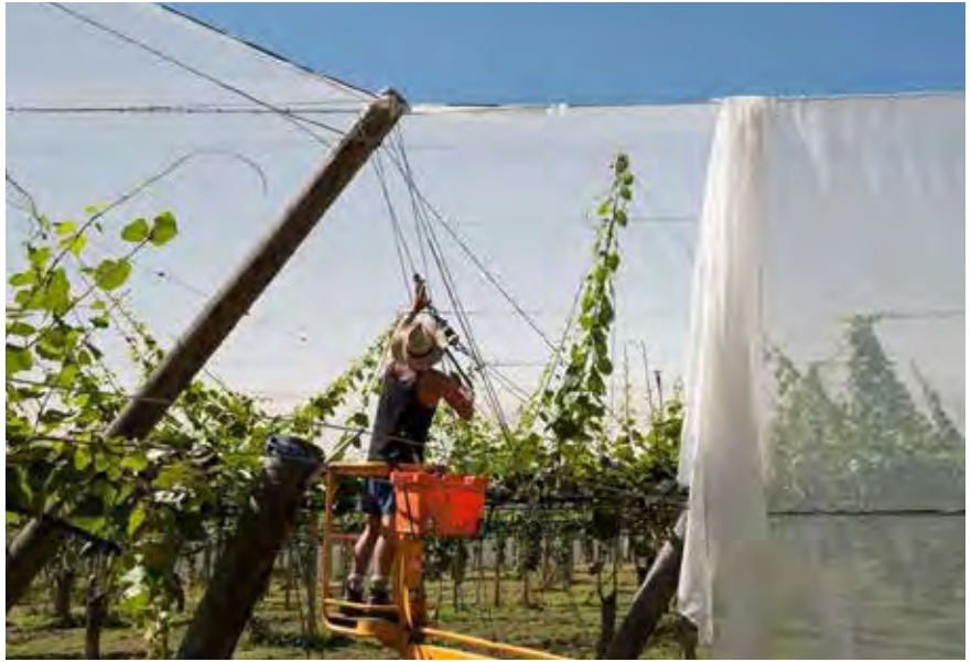
Right: The erection of hail netting over an orchard. In this instance the structure also has enclosed sides
