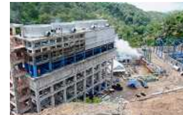
Site visit of Ulumba Geothermal Power Generation Plant
