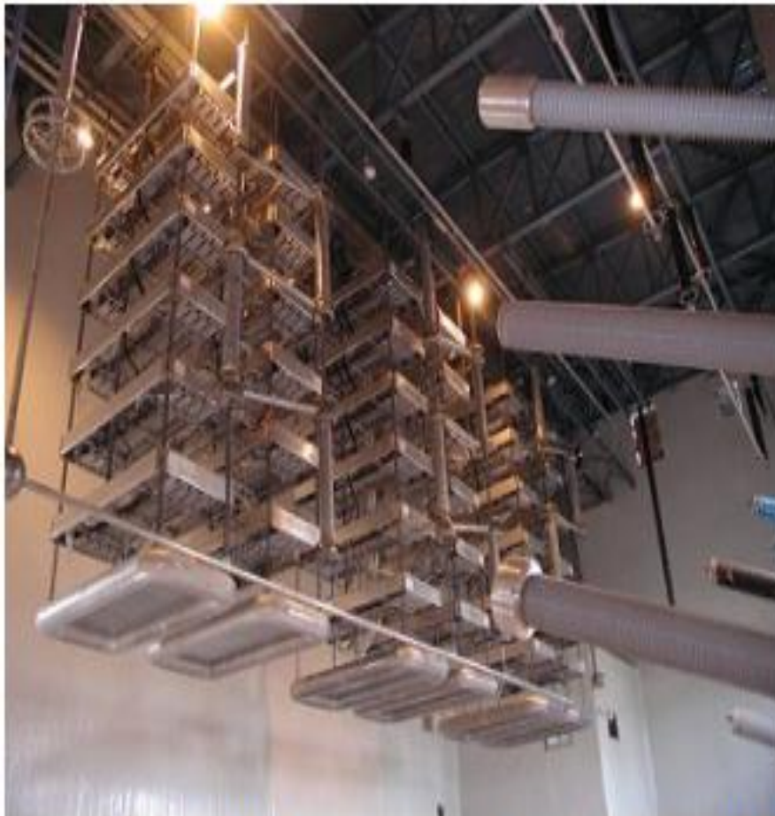
Suspended converter valves of a complete pole at Talcher
