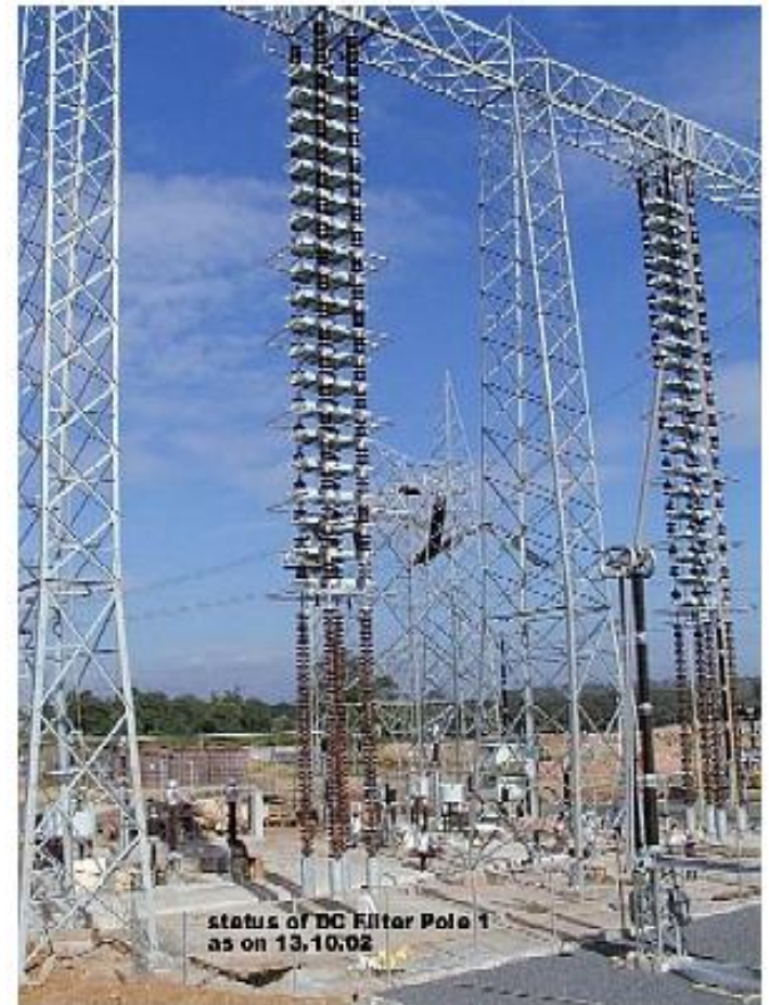
DC harmonic filters of pole 1, Talcher
