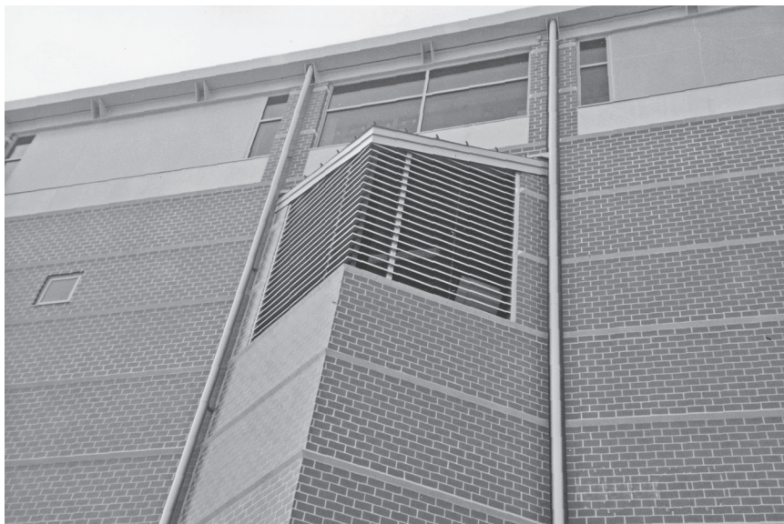
FIGURE 1.6. Air intakes for Monsanto Research Center in St. Louis are placed high to avoid street-level air pollution as a measure to improve indoor air quality.
