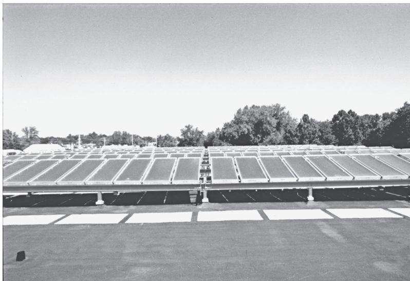
FIGURE 1.4. Solar collectors installed after the 1970s oil embargo were an opportunity to explore new technologies, but could not be justified on the basis of economics or life-cycle cost.
