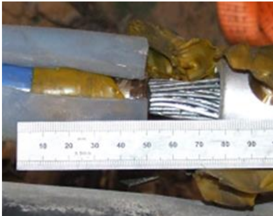
30 mm gap in insulation
