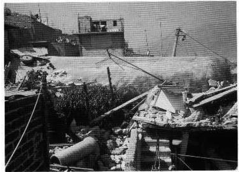
The cylindrical tank that flew furthest penetrated some 1,200 m into the housing area and crashed into a 2 storey house vacated one hour before.
