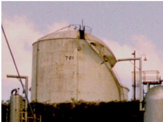
Local buckling of a tank
