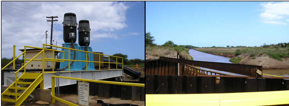
Figure 4. Drainage pumps and ditches located at the Mana Plain. (Photo: Joana Tavares, DAR)
