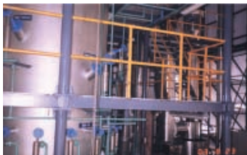
IISc Biomass Gasifier.
