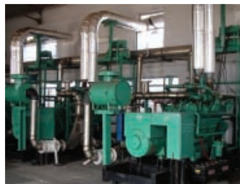
Gas Engines coupled to IISc Biomass Gasifier.
