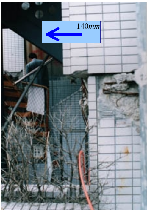
Photo.5 Failure of wall by slippage in elevator-shaft
