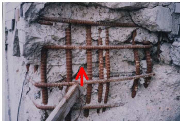
Photo.6 Slippage in the bottom connection of corner column on the first floor
