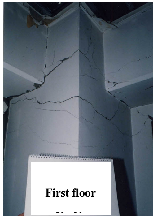
Photo.4 Shear failure in column-beam connection in second floor
