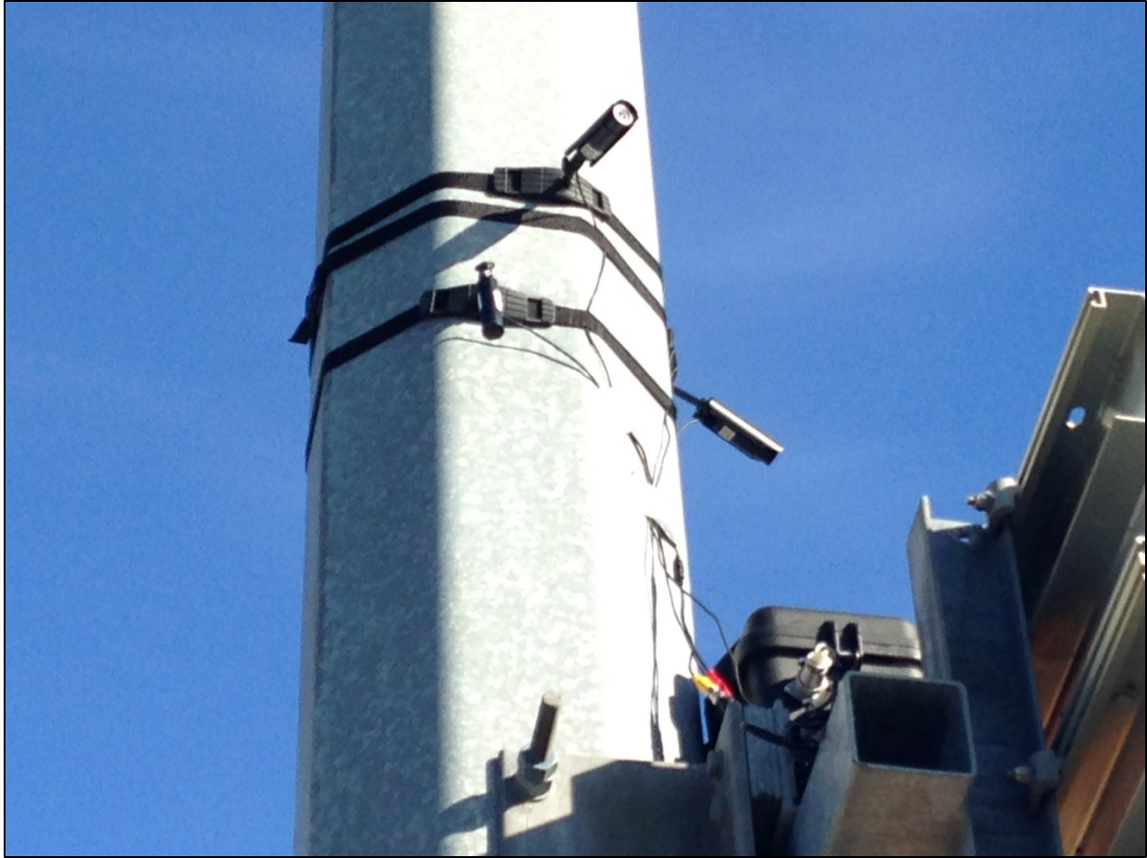
Figure 3.12: Video Camera Installation on Signal Pole
