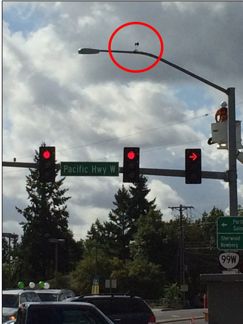
Figure 5.14: FLIR Trafisense Thermal Camera Placement Photo by Authors
