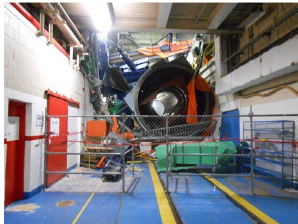
Figure 10 – Stator looking east
