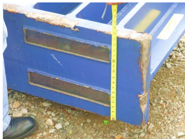
Figure 27 – Close-up of lower NW column
