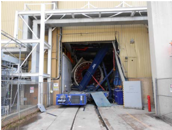
Figure 9 – Stator looking west
