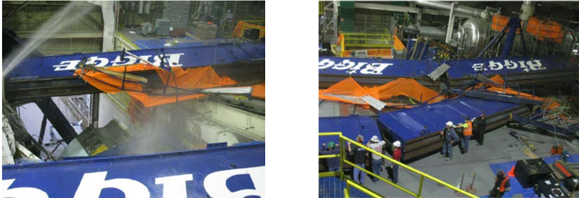
Figure 8 – Runaway girders after the collapse
