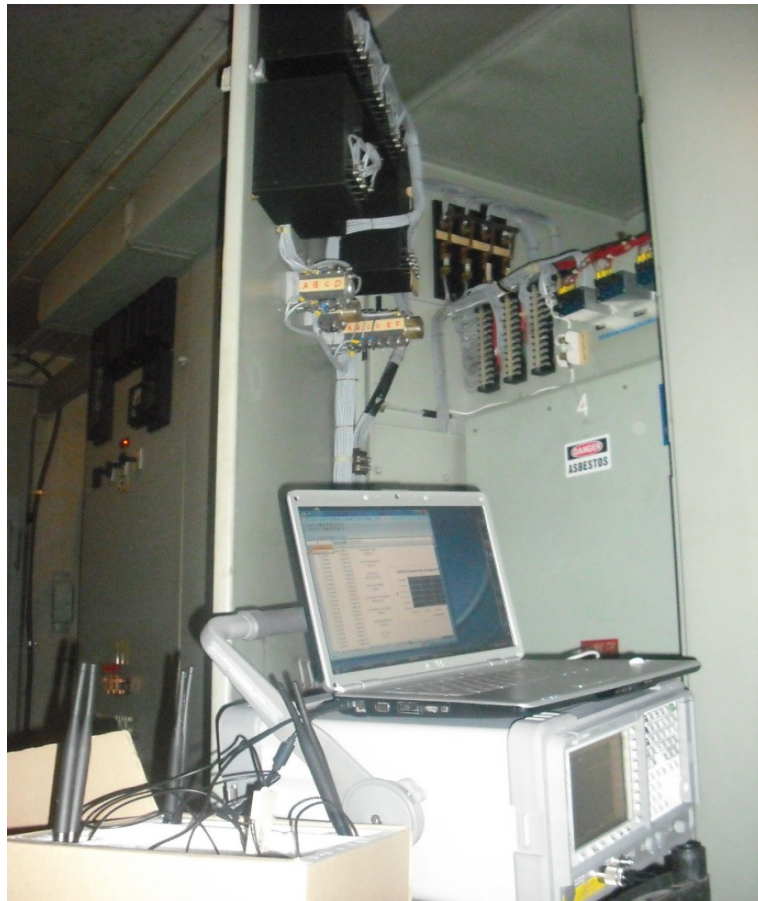
Figure 3-3 Test setup close to 13.8 kV CB at London Hydro distribution substation
