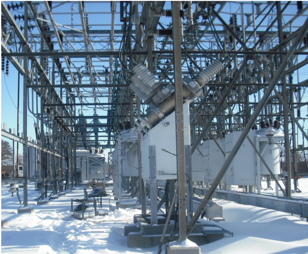
Figure 7-19 Wireless MU installed in switchyard of 27.6 kV substation
