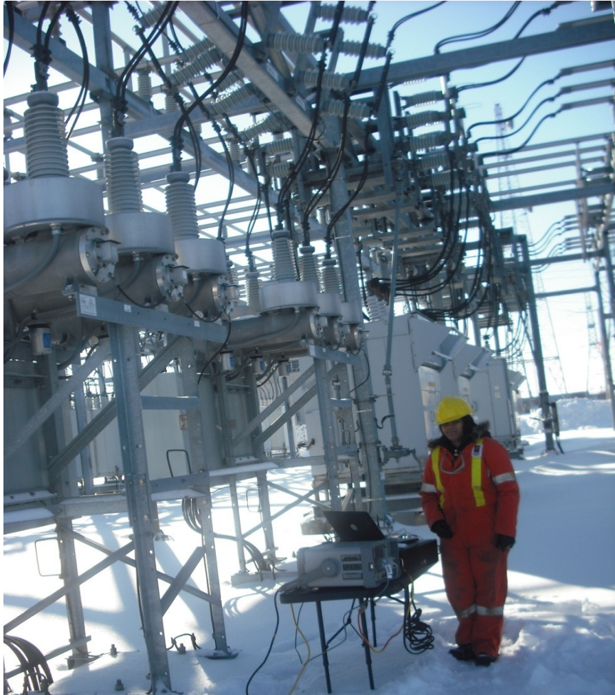
Figure 3-24 27.6 kV substation setup close to isolator switch in switchyard
