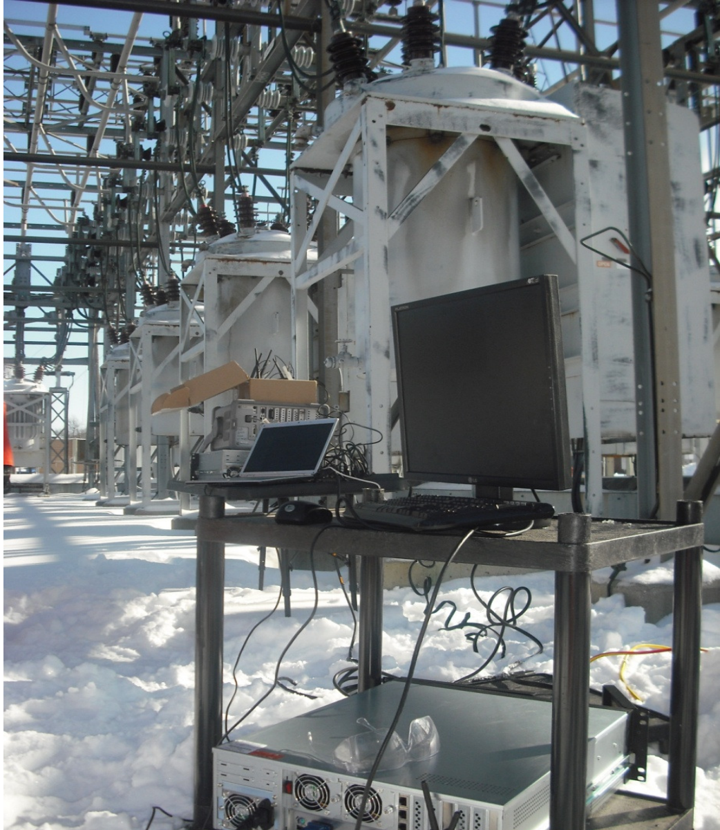
Figure 7-9 Wireless IED installed at 27.6 kV circuit breaker
