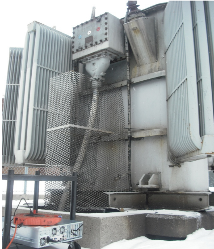
Figure 7-16 wireless IED installed close to 27.6/13.8 kV transformer in a substation
