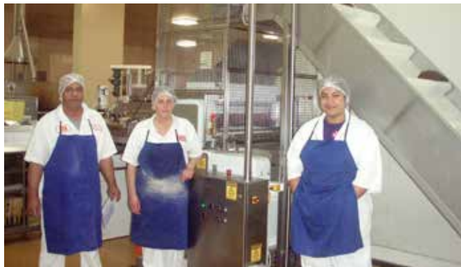
THIS PHOTO SHOWS SOME OF THE OUTCOMES FROM THIS PROJECT INCLUDING IMPROVED GUARDING ALONG THE SIDE OF A CONVEYOR, AN UPGRADED SWITCHBOARD (NOW STANDARD AT THE SITE) AND MESH GUARDING AROUND AN EXTRUDING MACHINE. WHEN THE DOORS ON THE MESH GUARDING ARE OPENED THE EXTRUDER IS AUTOMATICALLY ISOLATED (SWITCHED OFF).
