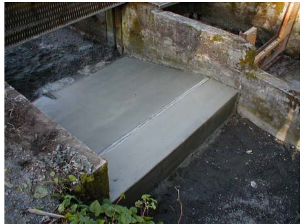
Figure WA9-1 Ramp Flume on the Sequim Prairie headgate Sequim, WA
