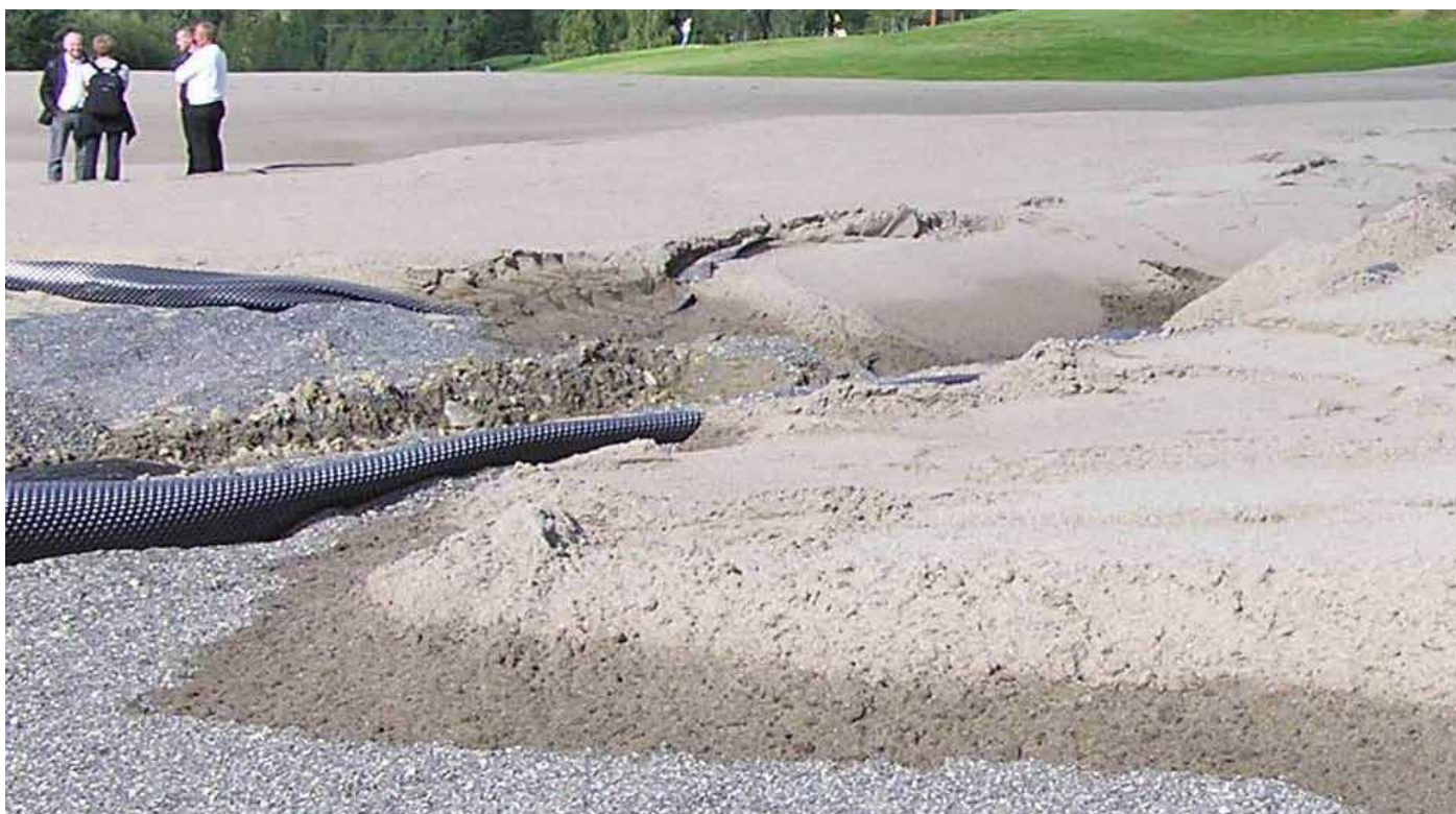
Photo 2. A perched water table is established by placing a fine-grained soil above a coarse-grained soil. Photo: Agnar Kvalbein.
