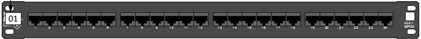
24-PORT PATCH PANEL
