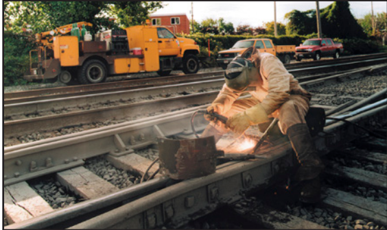
Railroad welding teams will appreciate the sizable air compressor, welding and 3-phase 240V power for grinders.
