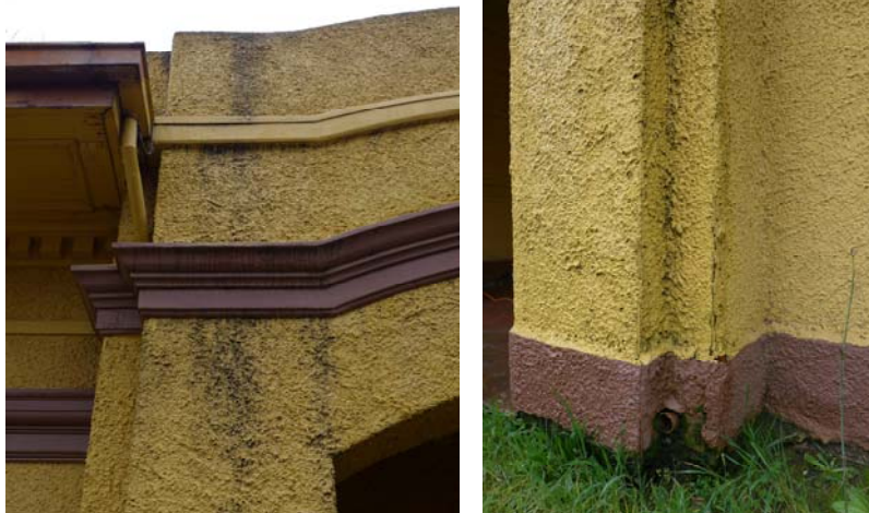
Figures 26 and 27. Gutters (left) and the downspout penetration (right) on the front façade.
