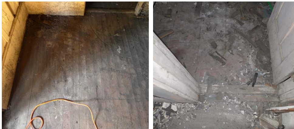
Figures 44 and 45. Wood flooring in the main room (left) and the vinyl flooring in the restroom (right).
