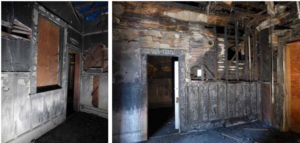
Figures 51 and 52. Wood trim in the office (left) and in the main room (right).
