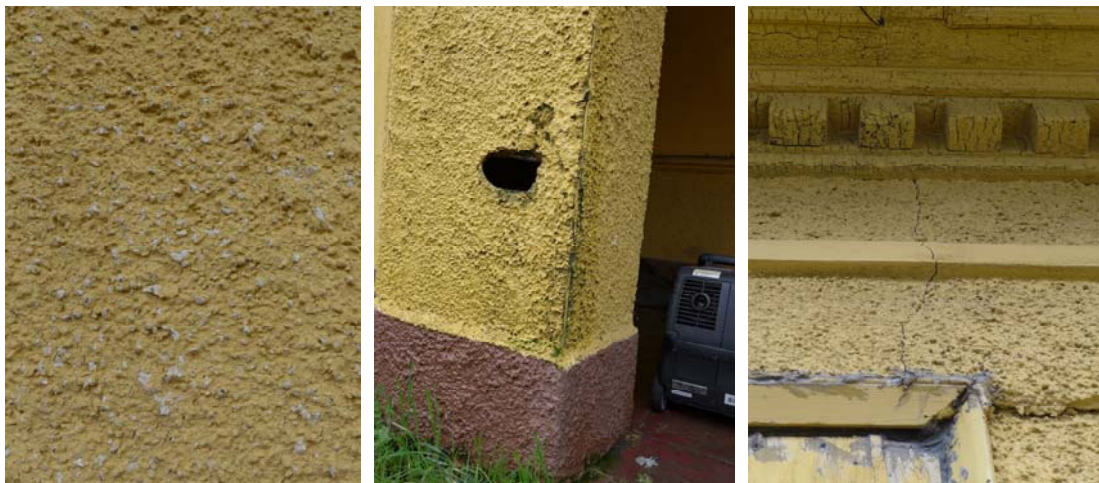
Figures 28, 29 and 30. (Left to right) Scaling paint, the hole on the front elevation, and cracking.
