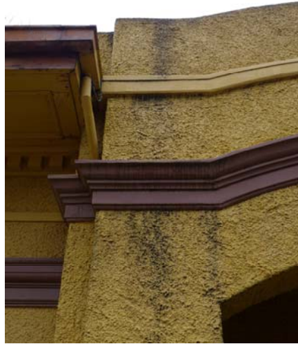
Figure 36. Black staining on the stucco.
