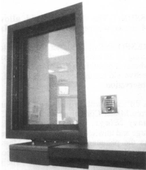
View from lobby of Master Control CCTV monitor and into the jail.
