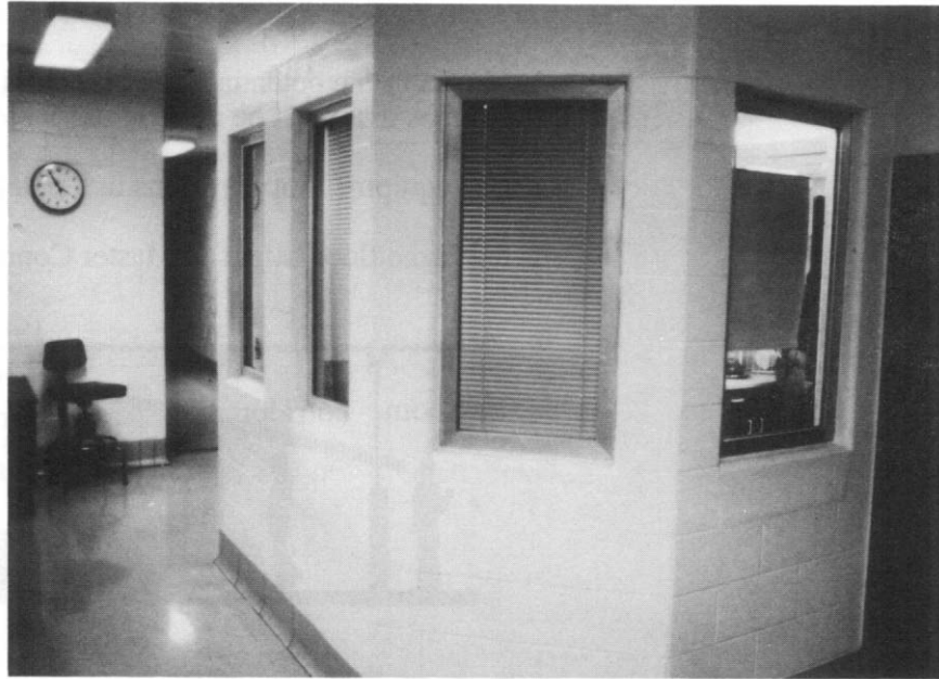
Blinds used by Master Control staff block view of staff by inmates, but defeat location and design of the space.
