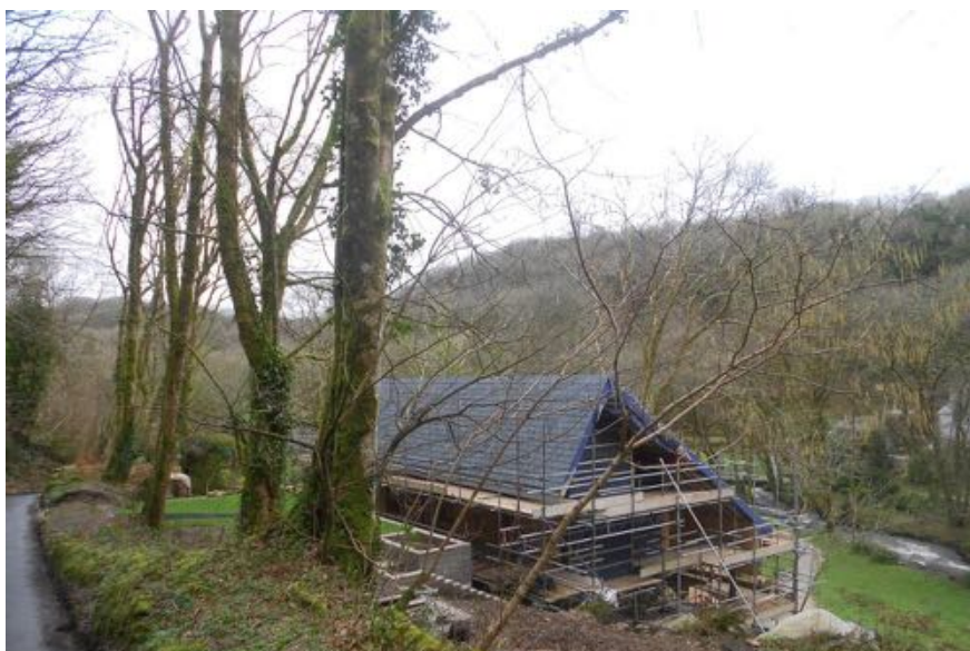
The roof is higher and different than that approved, plus an area of concrete hardstanding for vehicular access has been constructed.
