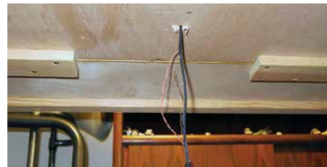
It doesn't look pretty right now under the table. You can see the damaged infrared sensor here. I wouldn't button everything up until you know for sure that the whole system works. The infrared sensor will be pushed up through the holes, and the tip of the sensor will be just below the track surface.
