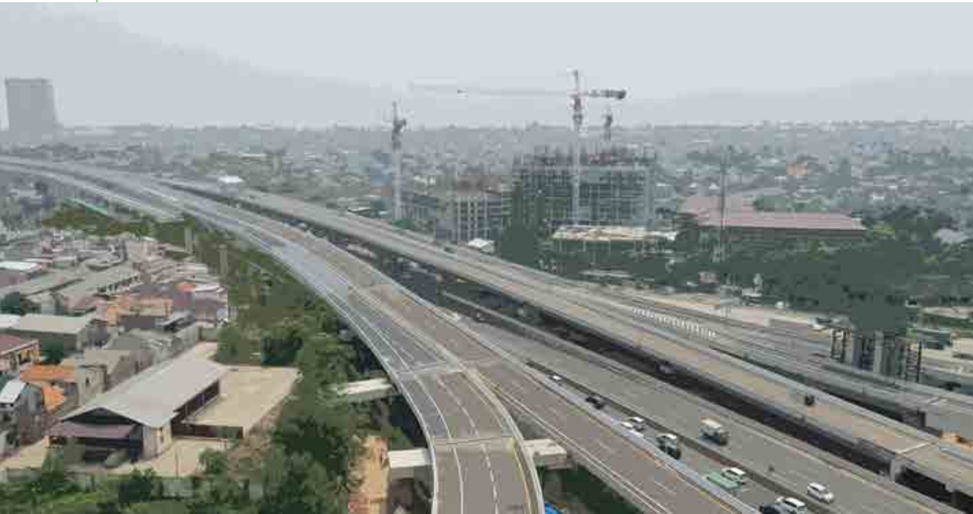
Jalan Tol Jakarta - Cikampek II Elevated / Jakarta - Cikampek II Elevated Toll Road
