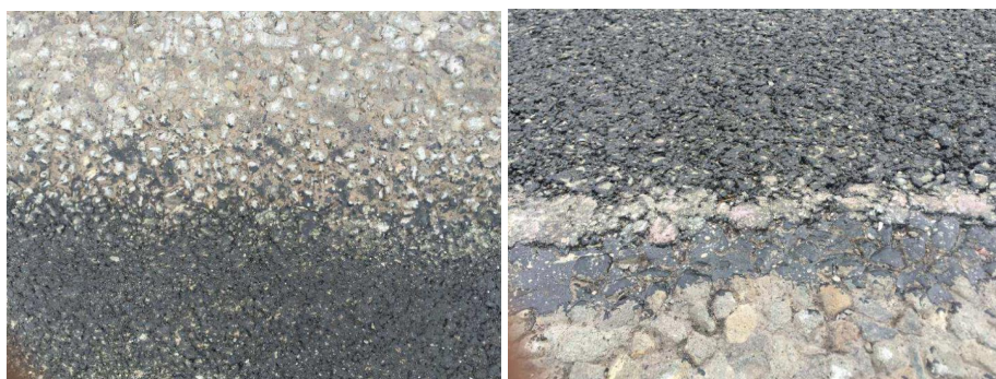
Figure 4: Joint Treated with Paver Mounted Heater (left) and Joint Untreated (right) - Area 9 Paver Mounted Heater Trials, 2016
