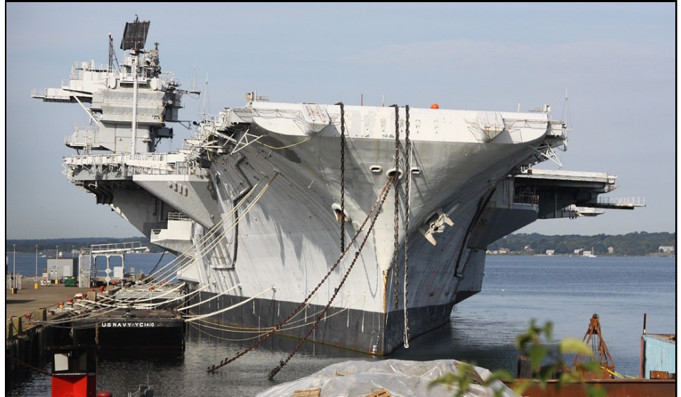
JMS conducted a survey of the aircraft carrier EX-SARATOGA (CV-60) to develop a preliminary towing and dismantling plan.
