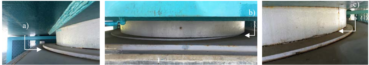
Figure 12. Information obtained from visual inspections carried out on the bearings of piers P2 and P3 of the Sado bridge.
