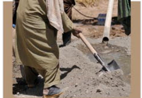
A Bowragay villager manually mixing concrete with a shovel used to build the casing around opening to the karez tunnel here June 5.
