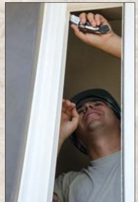
Sgt. Martin Mendoza, a Lake Elsinore resident with Headquarters and Headquarters Company, Maneuver Command, finishes the details of a window, June 10, as part of renovation efforts underway on Camp Roberts. Photo by Sgt. 1st Class Benjamin Cossel
