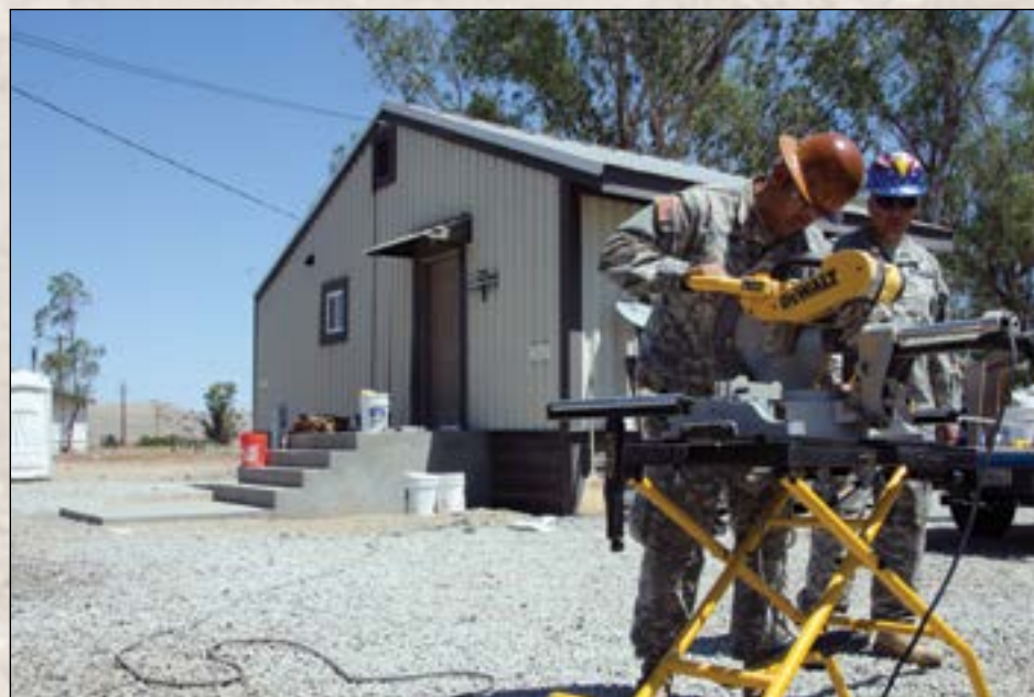
Los Angeles resident Spc. Jose Galban with the Camp Roberts Maneuver Training Command puts the finishing touches on one of four cottages recently remodeled and now open to military personnel and civilians alike. Photo by Sgt. 1st Class Benjamin Cossel
