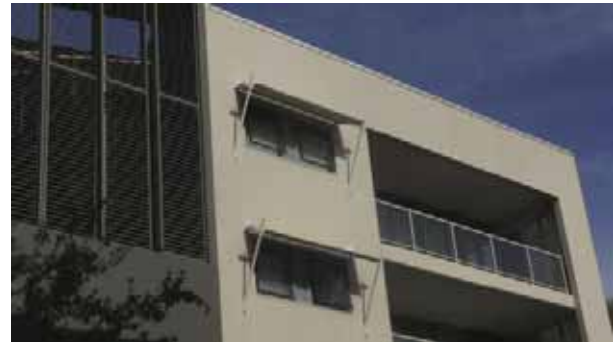
Photo K2-16 Horizontal sun shading over west facing windows protects from undesirable heat gain
