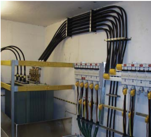
TFO-room in Trondheim, Norway.
