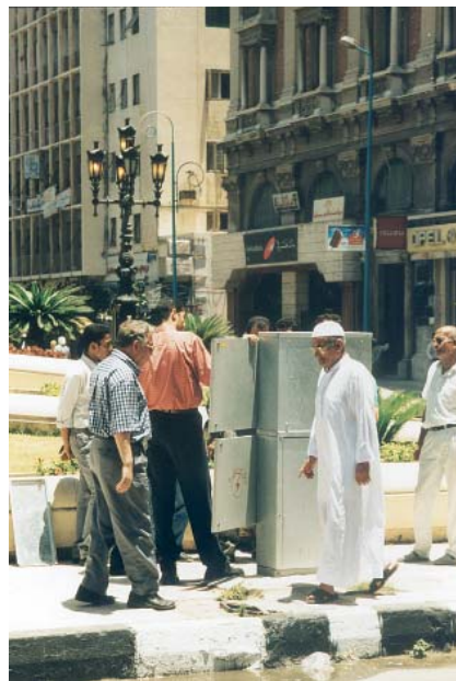
Cable distribution cabinet for street lighting box installed outside the Governor's Palace in Alexandria, Egypt.
