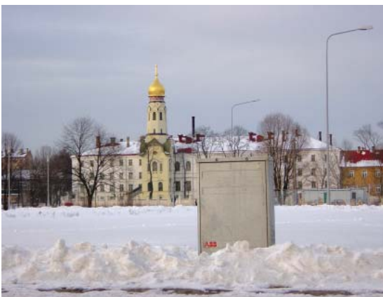
Lighting distribution board, Riga, Latvia.
