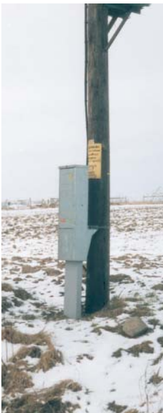
Pole-mounted cable distribution cabinet with cable duct to the ground.
