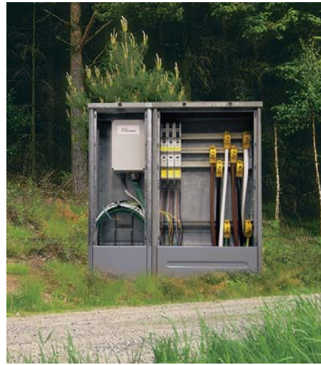
Cable distribution cabinets used as electricity and fibre optic networks (access network).
