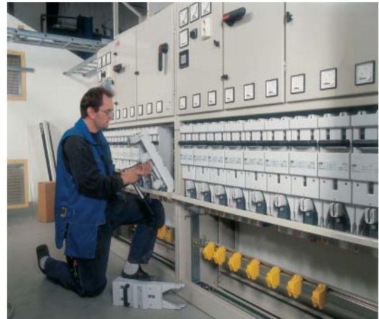
Busbars and devices are used in network and substation distribution boards.
