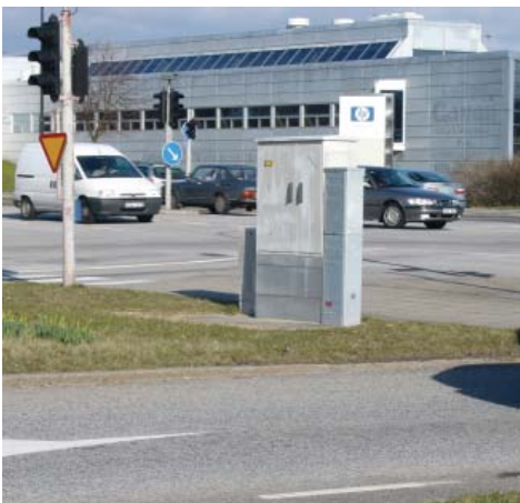
CDCM 420 for feeding and measuring of automatic equipment to traffic signals in Malmö, Sweden.
