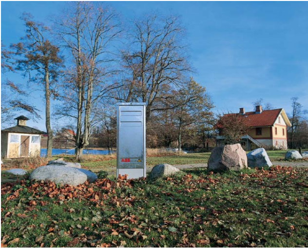
Cable distribution cabinet, Sweden
