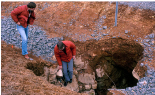
Figure 11. Cover collapse sinkhole along the ditch line of Tennessee Route 72, Loudon County.
