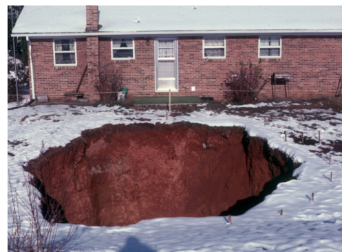
Figure 2. Sinkhole in a septic tank drain field in Hamblen County.
