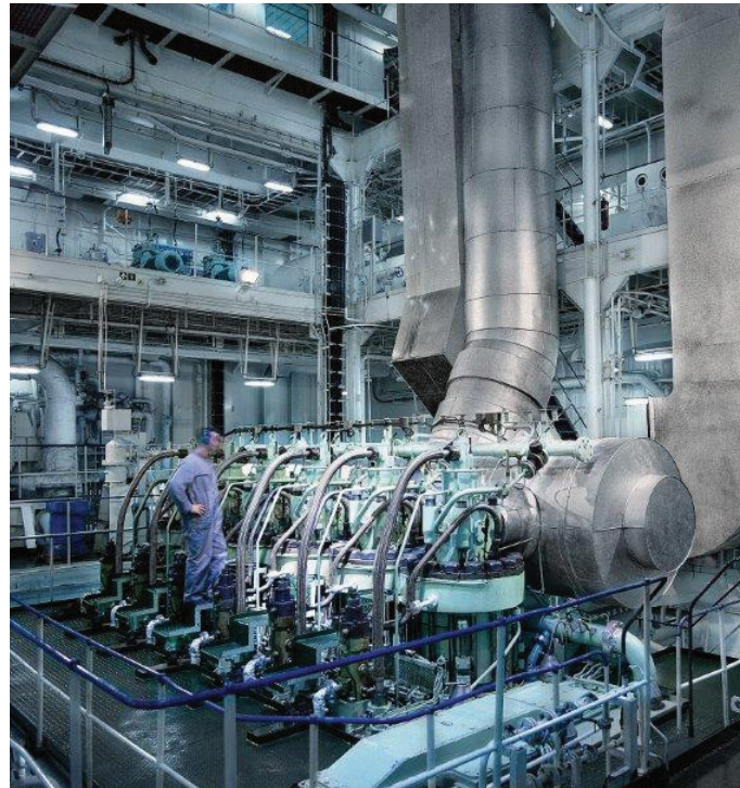
Example of hydraulics in harsh environment; Large 2 stroke marine engine with hydraulics valve actuation and fuel injection
