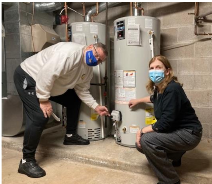
VF Rotarian Galen Powers (L) inspecting new hot water heaters with Serenity House Director Kayko Jarmusz
