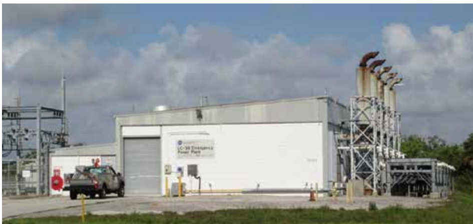
C5 Emergency Power Station - Oxidation catalysts were installed at the exhaust side of the engines in 2014 reducing CO emissions by >= to 70%.
