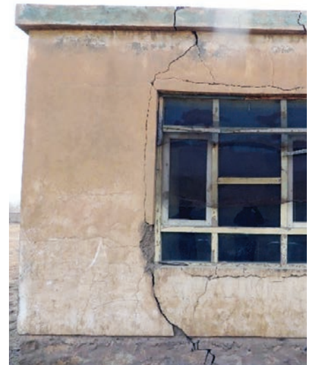
Large cracks in the wall of a school in Baghlan Province. (SIGAR photo)
