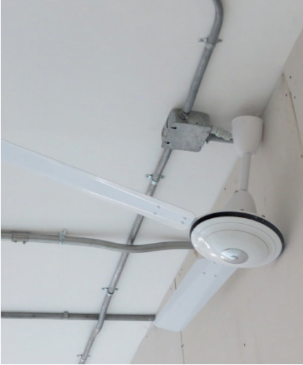
A suboptimal ceiling-fan installation at the Ministry of Interior headquarters building. (SIGAR photo)
