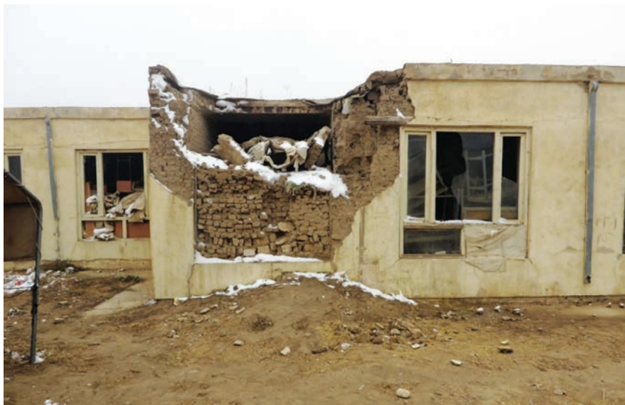
The wall and roof of a school in Baghlan Province that was damaged by an explosion. (SIGAR photo)
