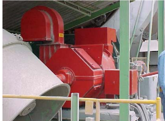
Figure 3 - 2 x 300 hp DC motor and drive train
