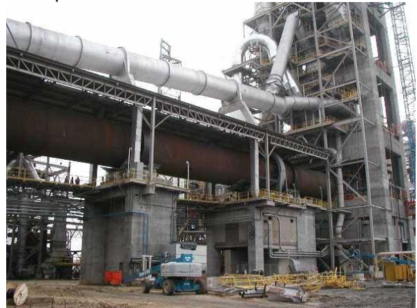
Figure 1- 6000 MTPD -3 support kiln powered by 1100hp AC drive
