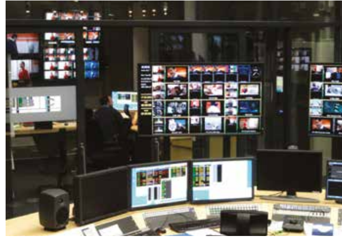
Broadcasting and production studios need access for multiple users and instantaneous switching for live broadcasts and updates.
