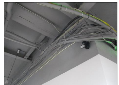
PHOTOGRAPH 12 TYPICAL VIEW OF MAIN BUILDING RISERS ON FIRST FLOOR OF BUILDING WITH BT COPPER AND FIBRE SERVICES
