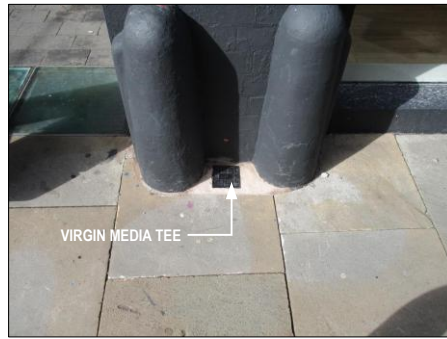
PHOTOGRAPH 5 EXISTING VIRGIN MEDIA DUCT AND TEE OUTSIDE BUILDING ENTRANCE ON GIBB STREET
