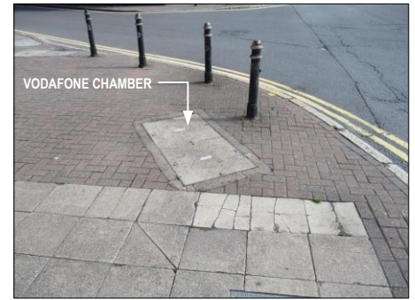
PHOTOGRAPH 6 EXISTING VODAFONE CHAMBER IN FOOTWAY AT JUNCTION OF HEATH MILL LANE WITH HIGH STREET DERITEND
