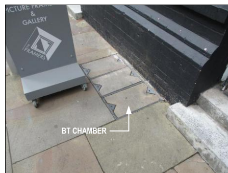
PHOTOGRAPH 2 EXISTING BT CHAMBER IN FOOTWAY ON GIBB STREET ADJACENT TO BUILDING ENTRANCE
