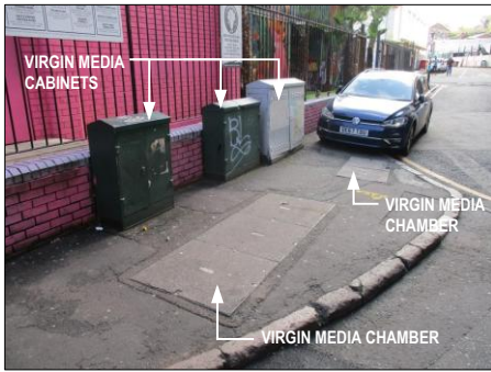
PHOTOGRAPH 4 EXISTING VIRGIN MEDIA CABINETS AND CHAMBERS IN FOOTWAY AT NORTH END OF GIBB STREET
