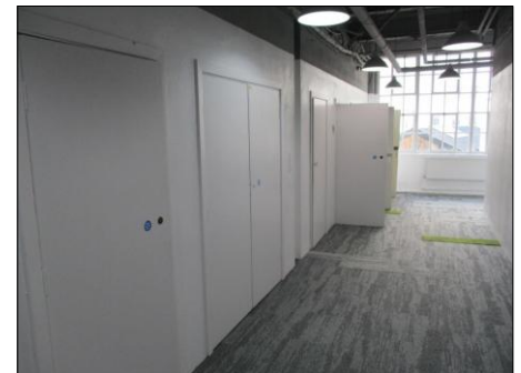
PHOTOGRAPH 9 TYPICAL VIEW OF MAIN BUILDING RISERS ON FIRST FLOOR OF BUILDING WITH BT COPPER AND FIBRE SERVICES
