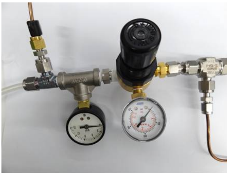
Figure 14.2 – Above is a N 2 Regulator Setup: Semitransparent tube on the left is from the 'WLM Purge' Port on the Analyzer. Copper colored tube on the top left
