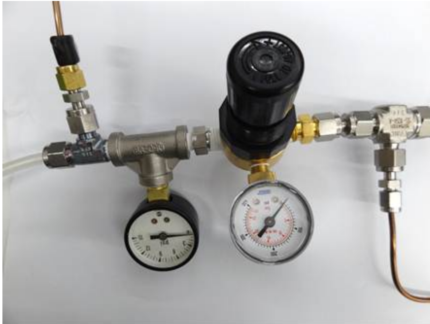
Figure 13 – Above is an N 2 Regulator: Semitransparent tube on the left is from the “WLM Purge” Port on the Analyzer. Copper colored tube on the top left comes from the Vaporizer. Copper colored tube on the bottom right goes to the the (N 2 or Dry Air) Gas Cylinder.
