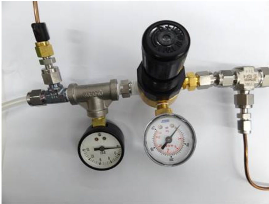
Figure 28 – Above is a N 2 Regulator Setup: Semitransparent tube on the left is from the ‘WLM Purge’ Port on the Analyzer. Copper colored tube on the top left comes from the ‘Purge’ and the ‘Sample’ ports on the Vaporizer (from the Vaporizer Switching Valve). Copper colored tube on the bottom right goes to the the (N 2 or Dry Air) Gas Cylinder.
