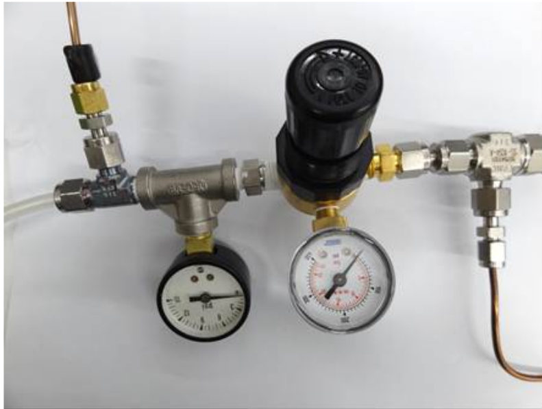
Figure 12.2 – Above is an N 2 Regulator: Semitransparent tube on the left is from the ‘WLM Purge’ Port on the Analyzer. Copper colored tube on the top left comes from the ‘Purge’ and the ‘Sample’ ports on the Vaporizer. Copper colored tube on the bottom right goes to the the (N 2 or Dry Air) Gas Cylinder.
