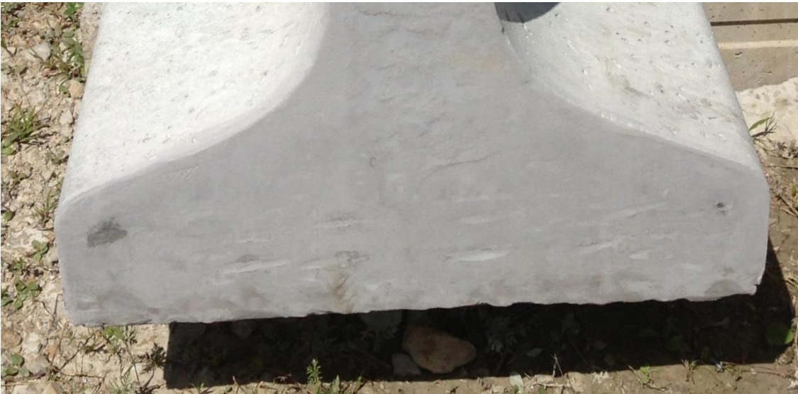
Figure 52. BD08506 before application of BASF Hydrozo 100
