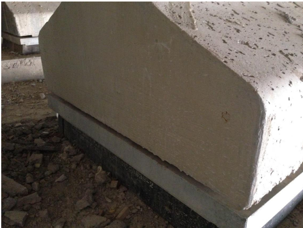
Figure 72. Poor field performance of Sikagard 62 on bridge beams
