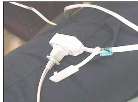
Electrical cords daisy-chained
