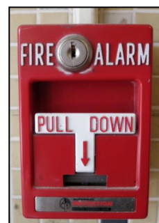
Fire alarm pull station
