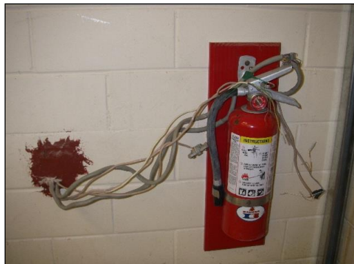
Blocked fire extinguisher
