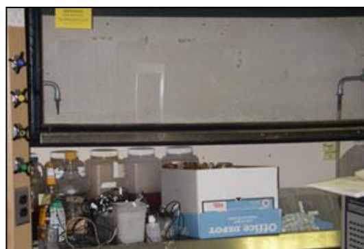
Improper storage in a fume hood
