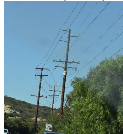
Example of overhead powerlines
