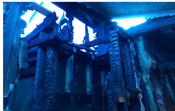
Structure fire that occurred in Laguna Beach
