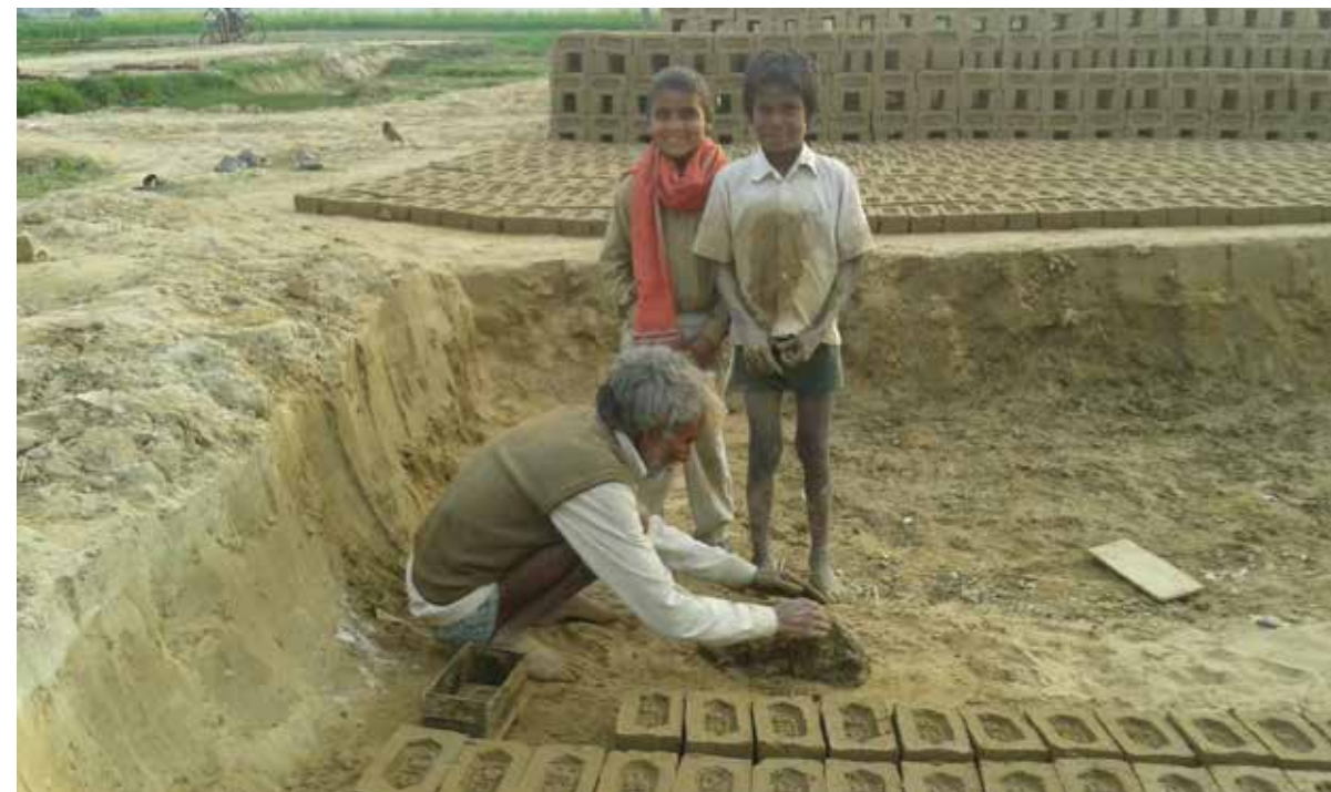
Opposite page, top left: foundation trench with baked brick and stabled cement mortar. Top right: baked brick external walls upto cill level. Below left: building the adobe walls. Below right: red sandstone slab chajjas. This page left: making of adobe. Below left: exposed brick arches in verandah. Below right: eucalyptus rafters nailed to jamun wood wall plates. Far below right: eucalyptus rafters at 1 foot spacing
