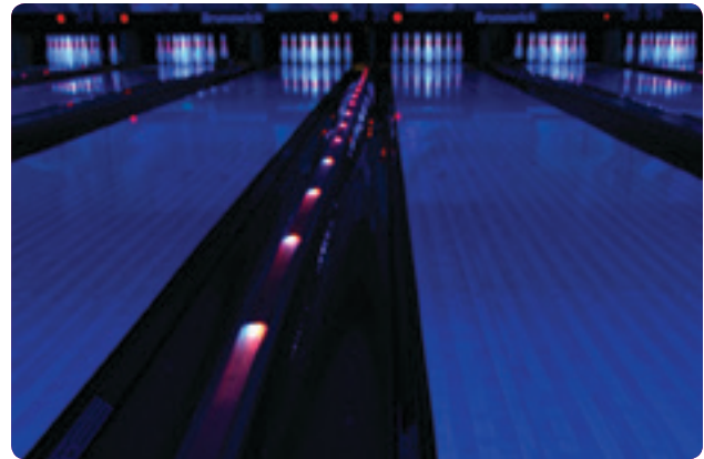
Lightworx Division Lighting System
