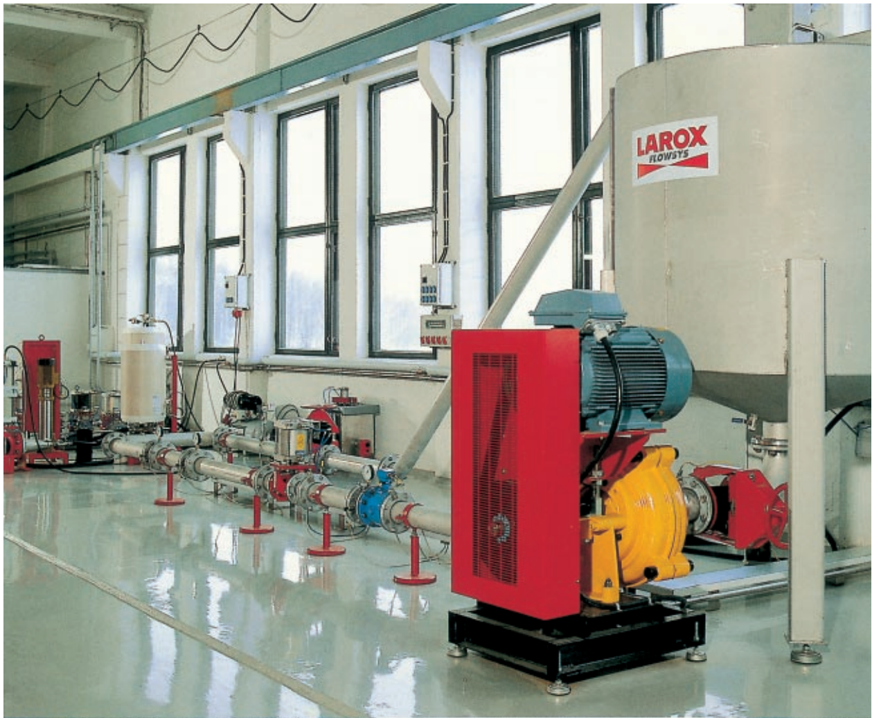
Closed pumping and circulation system in Larox Research Center.
