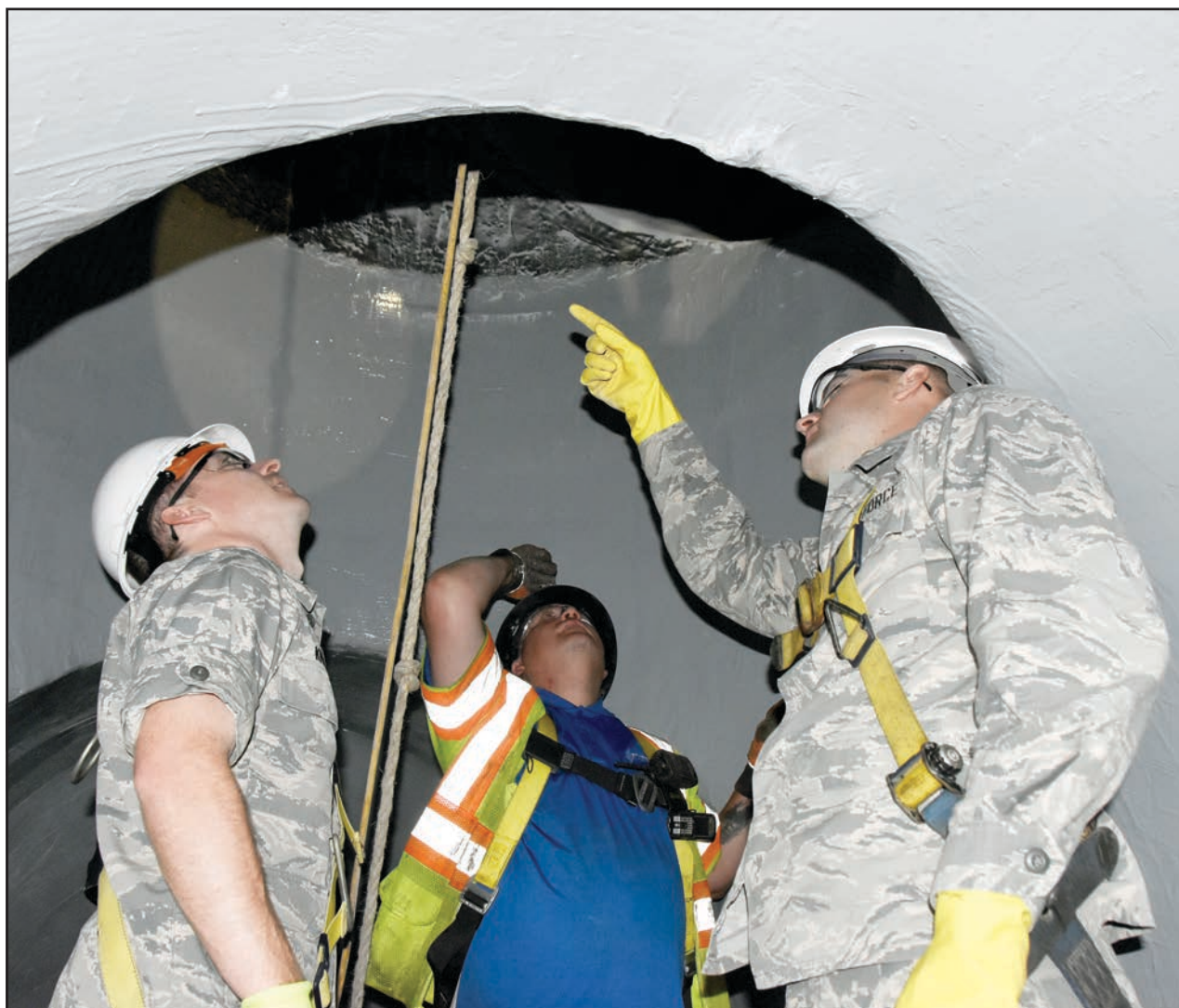
Maj. Michael Knauf, from left, Dusty Pickens and 2nd Lt. Adam Doyle conduct an inspection of raw water pipes that were recently lined with a fiber-reinforced polymer, Sept. 23 at Arnold Air Force Base. (U.S. Air Force photo by Bradley Hicks)
