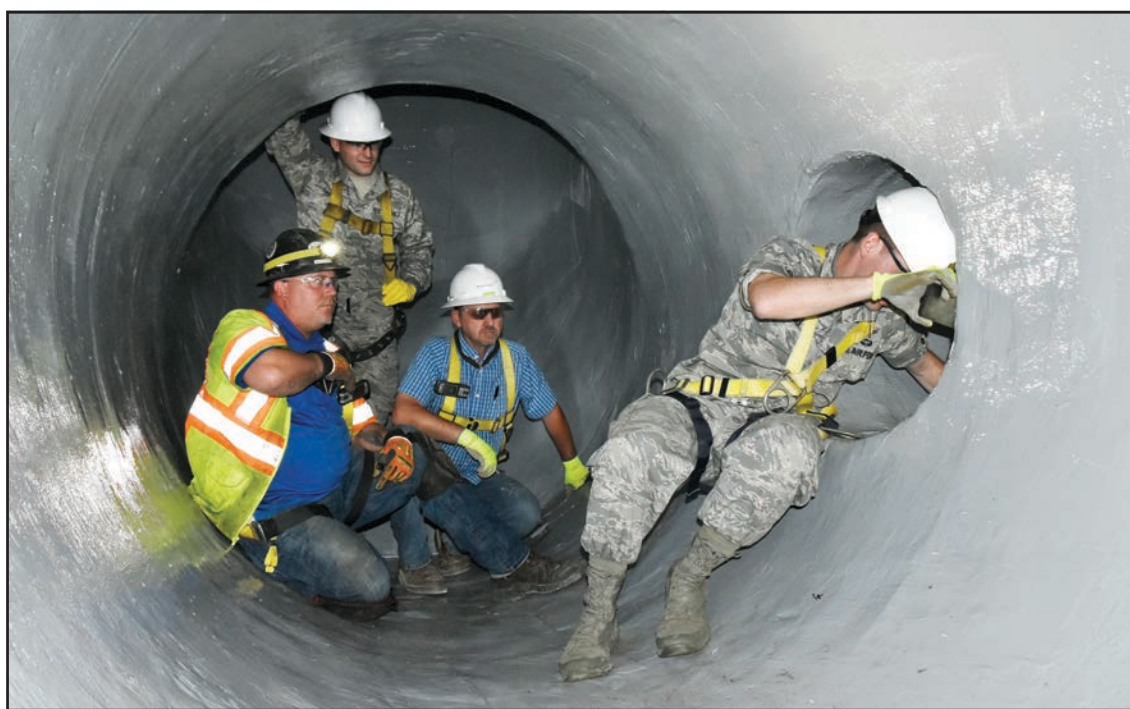
Dusty Pickens, from left, 2nd Lt. Adam Doyle and Andy Crum look on as Maj. Michael Knauf exits a 30-inch pipe in the raw water pipe system at Arnold Air Force Base. The group conducted an inspection of pipes recently lined with a fiber-reinforced polymer, Sept. 23. (U.S. Air Force photo by Bradley Hicks)
