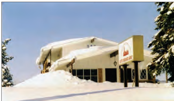
MBMA-sponsored research at Rensselaer Polytechnic University has improved our knowledge of how snow drifts across low-slope gable roofs as shown in this photo.
