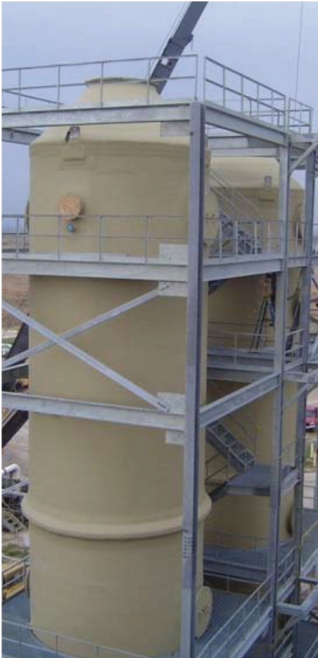
BELCO manufactured two, 68 foot tall FRP columns for Woodward Iodine
