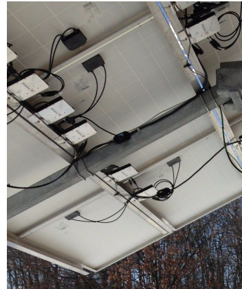
Fig. 2: Microinverters located on backside of panels
